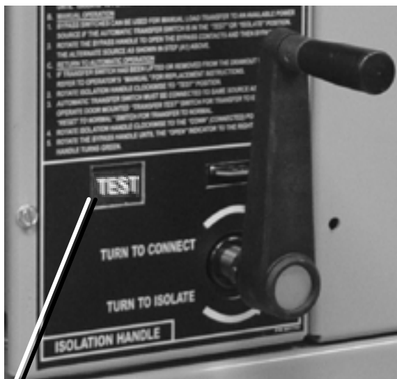
position window CONN TEST ISOLATE counterclockwise – draws out the transfer switch
